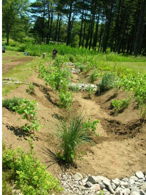
Figure 5 - Bioswale (Trinkaus Engineering, LLC)
